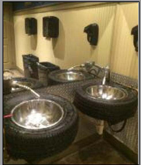
Sinks at Ford Restaurant, Florida
